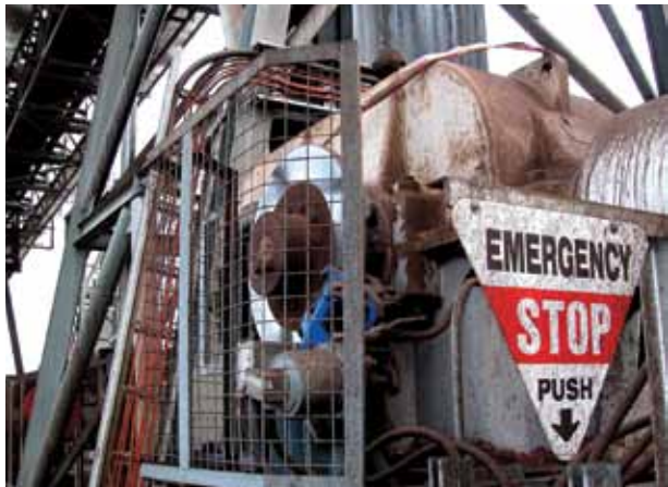
Twiflex GMR-SH spring-applied hydraulic released brake units fitted to a power station conveyor in Victoria, Australia.
