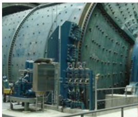
Twiflex VMS-DP brake calipers (with pedestals) plus a hydraulic power pack installed on a 22.5 MW SAG mill, 11.6 m dia. x 13.7 m long, at a copper mine in Sweden. The 8-off VMS-DP brakes produce 38 MNm braking torque and can stop the mill with the 1375 Mg full process charge in less than 2 seconds.
